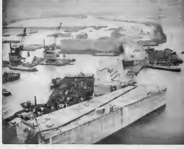
WHEN THE LAST caisson was shoved in place it joined three others in the formation of a new dike at Ouwertrek. Willow "matresses" float near the caissons. The area to the right of the dike is all flooded land.
